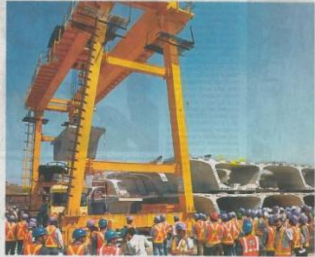
Viaduct segments for Hyderabad Metro Rail project being manufactured at Quthbullapur casting yard in Hyderabad on Tuesday | enr.in
