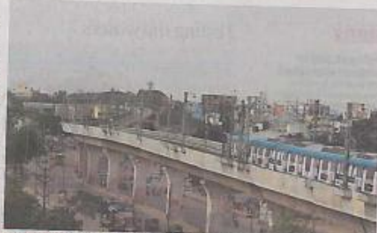
CRUISING AHEAD: Out of the total 72 km, foundations on 39 km, pillars on 36 km and viaduct on 47 km have been completed so far. (A. Srinivas)
