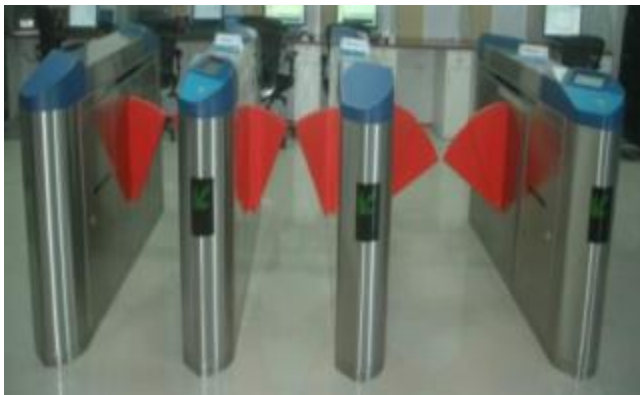
Automatic Fare Collection gates
